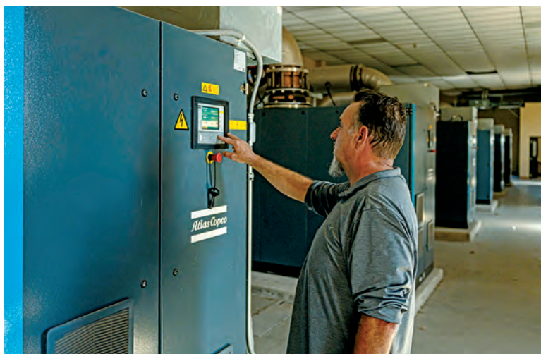
Shannon Bailey, shown checking on the plant's Atlas Copco turbo blower, fosters an environment where every team member takes responsibility for treatment performance and facility appearance.
