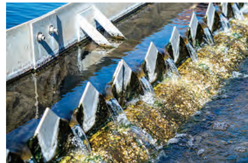
Final clarifier effluent from the activated sludge process is discharged to Wheeler Lake, an impoundment of the Tennessee River.
