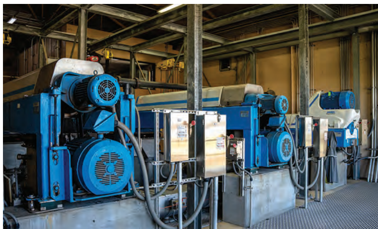
The Dry Creek plant's three Andritz centrifuges dewater biosolids to 26-27% solids.
